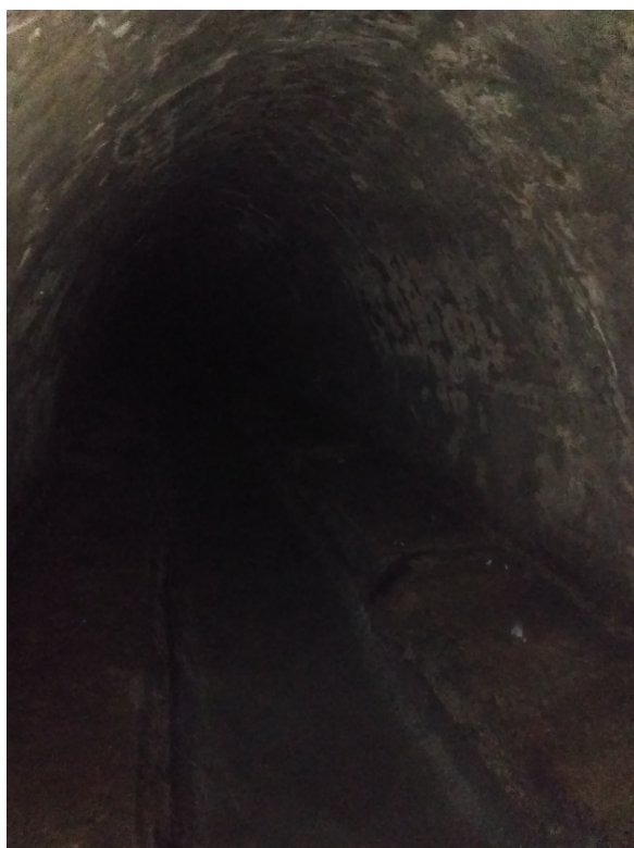
Photo 1 – Sewage collector on Akademika Sakharova Street (Lviv)
